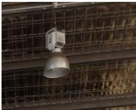
Non illuminated High Bay lighting fixture.
